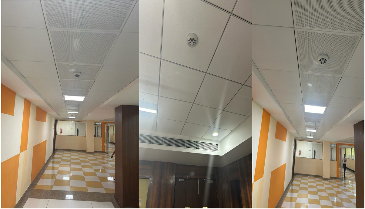
Picture 3: Smoking alarms and detectors installed in MUJ to ensure No Smoking in the campus
